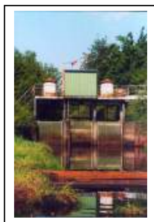
Station de pompage
